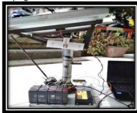
Gambar 4.3 Tampak Samping Panel
